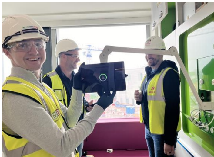
David Flood from Oneview's Dublin office overseeing the Oneview installation in Children's Hospital Ireland's "Mock Room"
